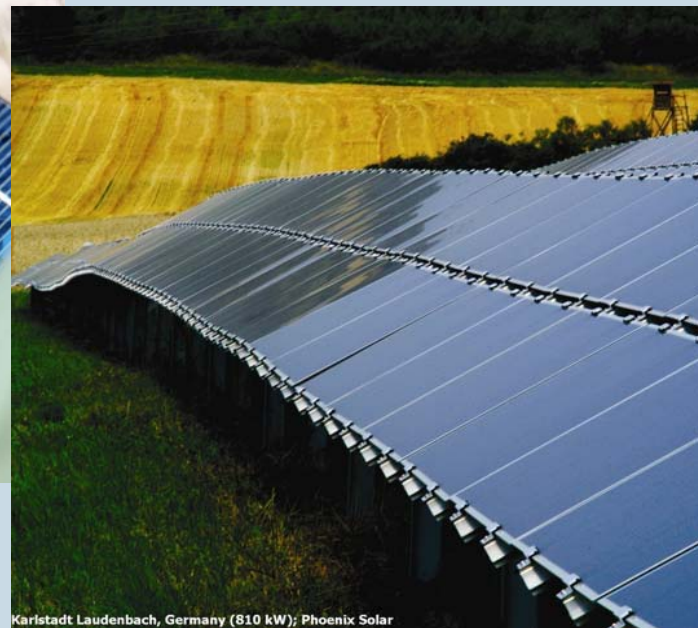
Karlstadt Laudendach, Germany (810 kW); Phoenix Solar
